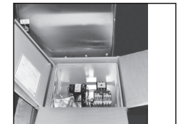
Inside the Control Panel enclosure (if supplied).
