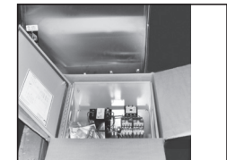
Inside the Control Panel enclosure (if supplied).
