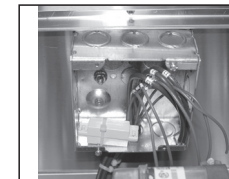
Inside the junction box.
