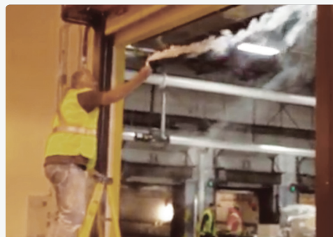
When the air curtain is not operating, the smoke flows through the opening and rises.
